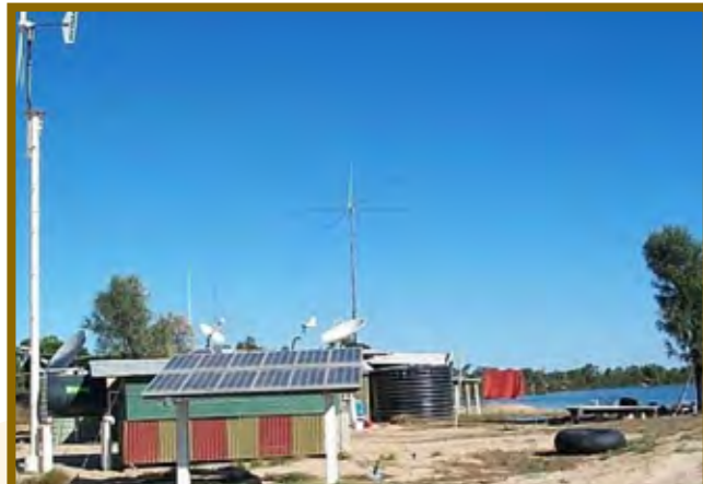
The Bradley's home and business are now partially wind and solar powered.
